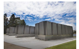
Solution 250 kW to MWs
